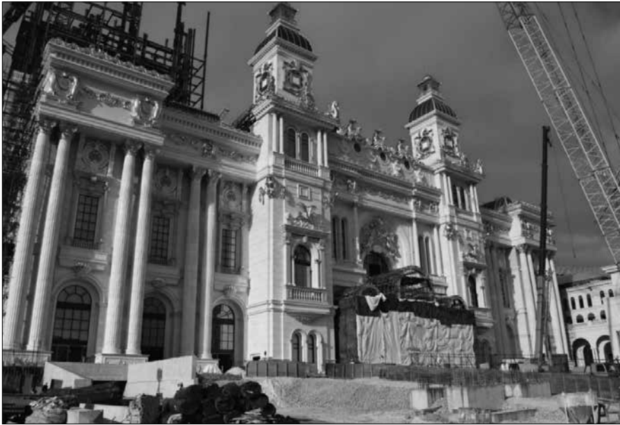
Figure 1. The Imperial Pacific Resort Hotel (pictured under construction) is part of a $7 billion resort and casino development with ties to the PRC on the CNMI island of Saipan
